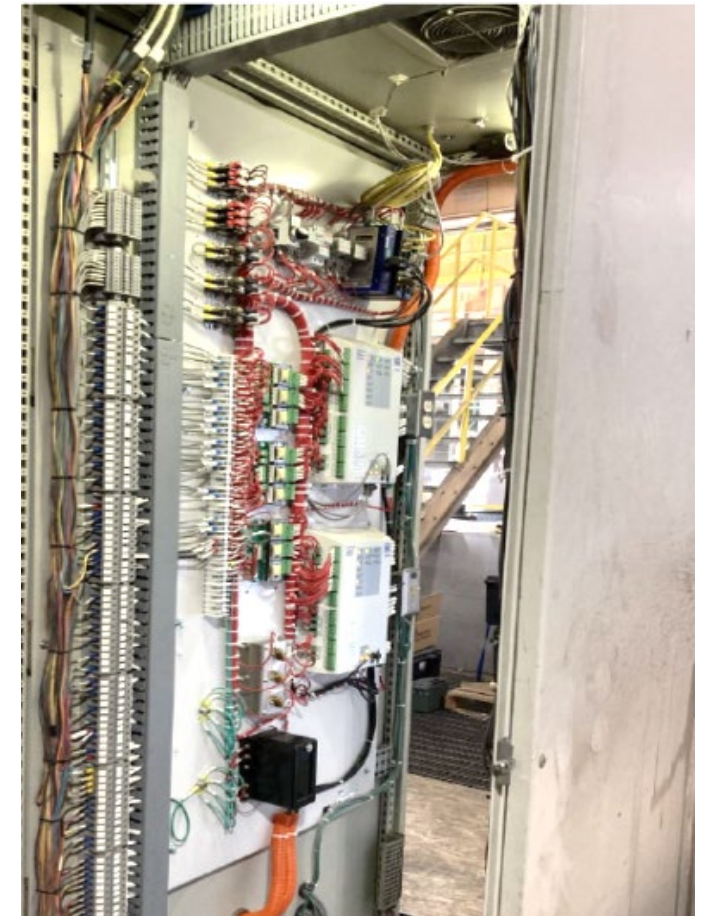
DECS-2100 ECM-2 Control Panel
