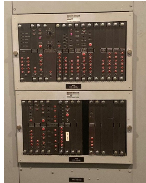
Old Busfed Control Panel
