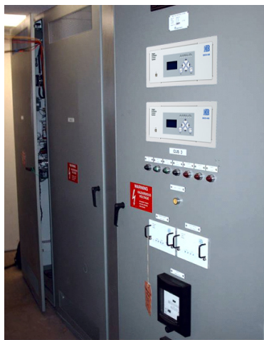
Figure 1: New Alterrex Digital Voltage Regulators Mounted in Cabinet
