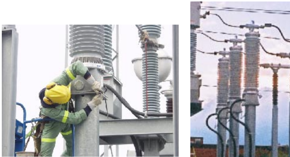
Figure 12: Installation of optical voltage and current sensors at a gas-turbine generating station.
