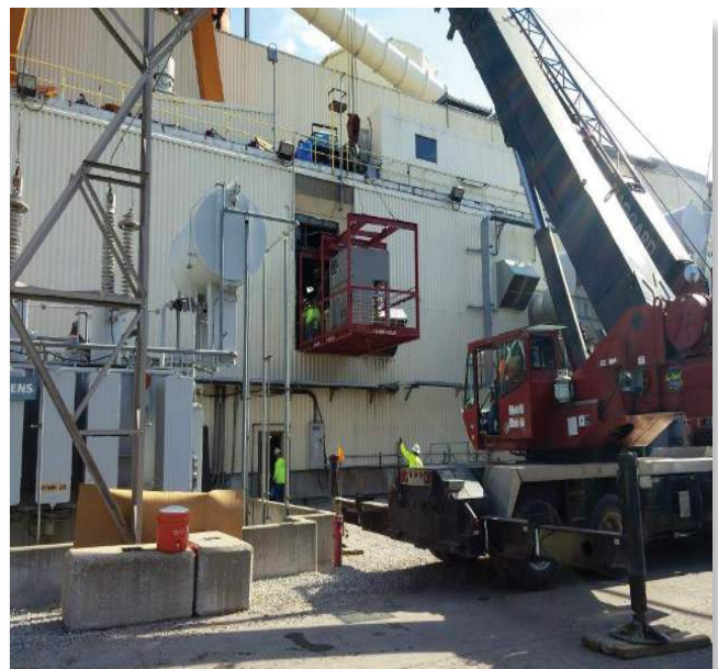
Figure 2 - Loading the new DECS-2100 into the facility
