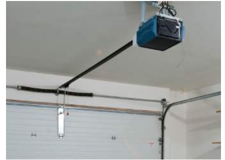
Garage Door Controls
