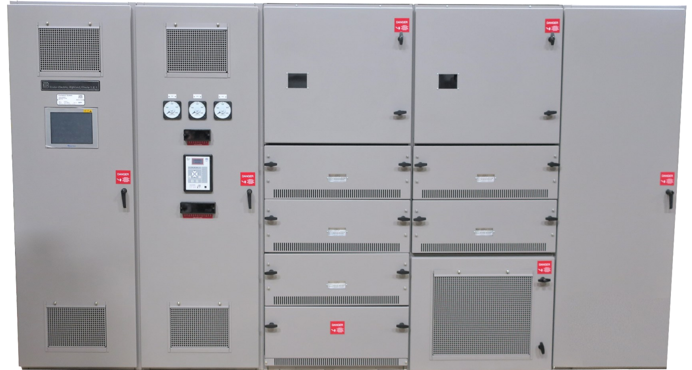
DECS-2100 System with N+1 redundancy rated for 3,100 Adc and a Basler BE1-11
